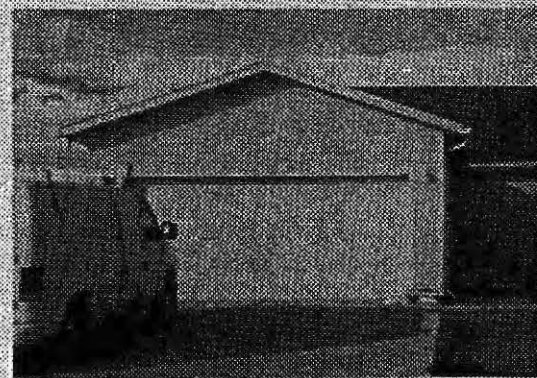
Example of a roof pitch that is too shallow
